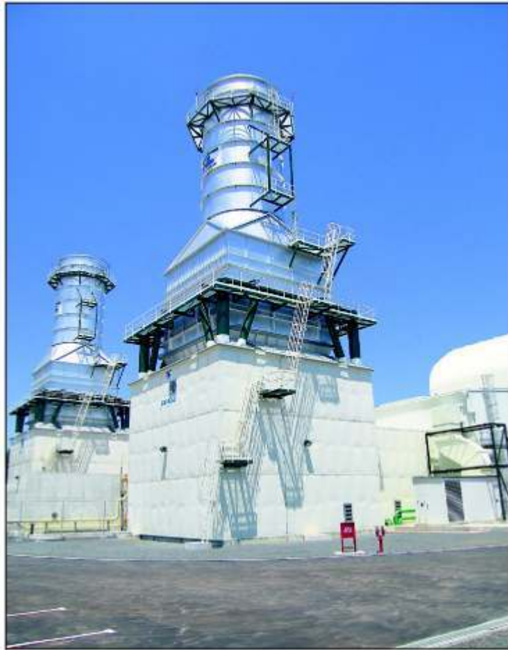
Powering up: Transfield Services is operating in the Kemerton estate.
